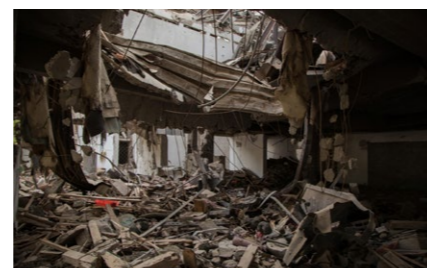
Above: Destroyed buildings like these former homes, schools and businesses have become the norm for many families living in Yemen as the destruction continues to escalate.
